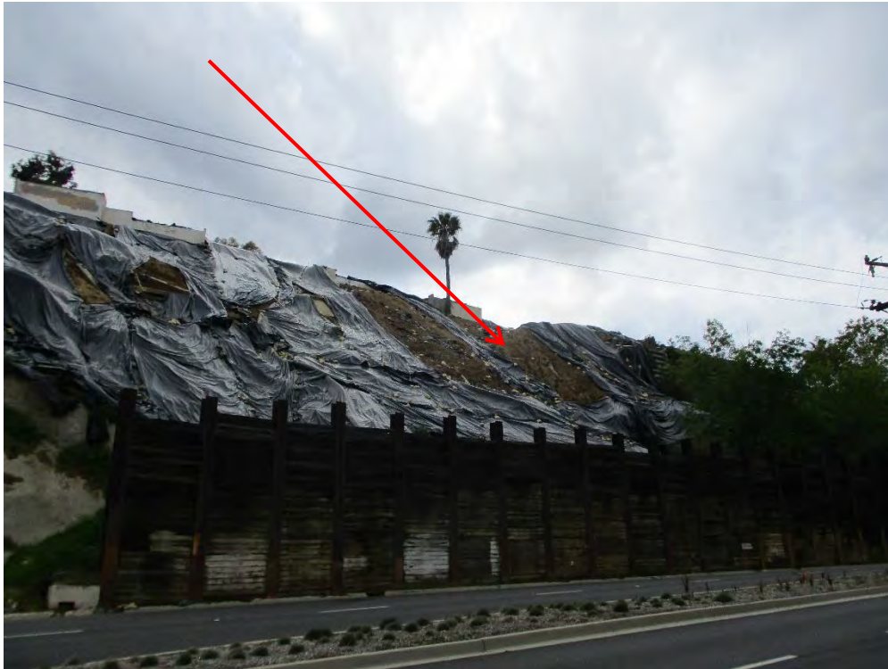
Garvey Ave - Gaps in Slope Plastic Sheeting Requiring Repair
