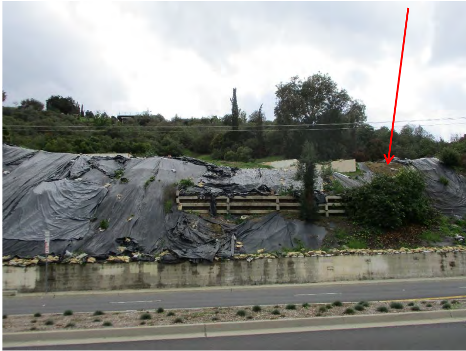
Garvey Ave - Gaps in Slope Plastic Sheeting Requiring Repair and Deteriorated Sheeting Requiring Replacement Still Present
