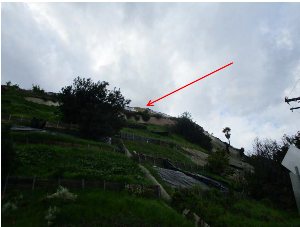
Garvey Ave - Gaps in Slope Plastic Sheetting Requiring Repair
