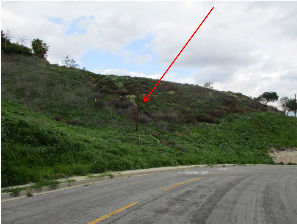
Slope View from Abajo Drive Looking North – Plastic Sheetting Remnants Still Present
