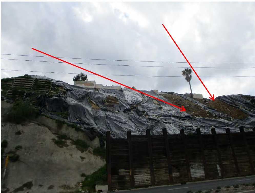
Garvey Ave - Deteriorated Plastic Sheeting Still Present
