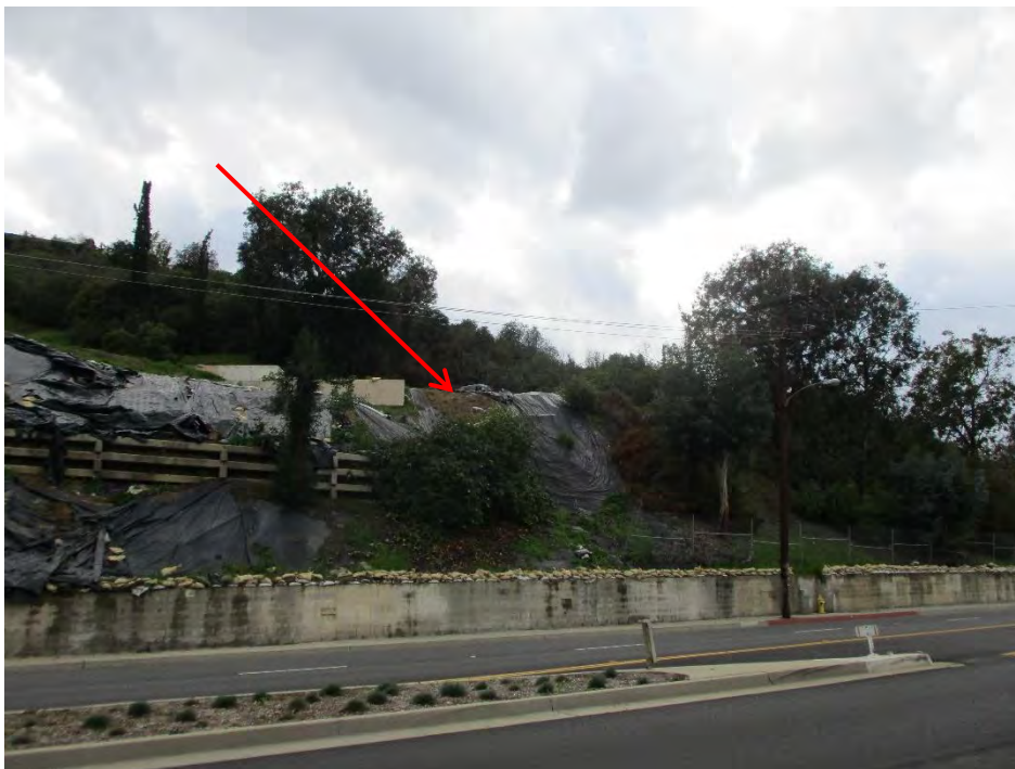
Garvey Ave - Gaps in Slope Plastic Sheeting Requiring Repair and Deteriorated Sheeting Requiring Replacement
