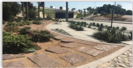
Washington Bl Widening and Reconstruction Project ($30M): The project included widening and reconstruction of 2.7 miles of Roadway, Traffic Signals, Street Lighting, Landscape, Improvements at I-5 and at 710 Freeways ramps. The project was federally funded and was managed in compliance with Caltrans LAPM.
