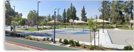
Almansor Park Improvements Project ($2.5M): This project was at Almansor Park in the City of Alhambra and included construction of new basketball courts, restroom facilities, shade structure, new drainage systems, new lightings, and updated landscaping and irrigation, and PCC walkways.
