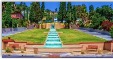
Cascades Waterfall Renovation Project ($.6M): This project included the renovation of the Cascades Waterfall landmark in Monterey Park, which included lighting, plastering of the fountain, painting, ADA improvements, PCC walkway improvements, and landscaping.
