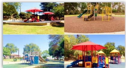
Citywide Parks Improvement Project ($6.5M): This project included installation of park equipment (playground, picnic shelters, benches), construction of ADA improvements, and various PCC improvements at 13 parks in the City of Monterey Park.
